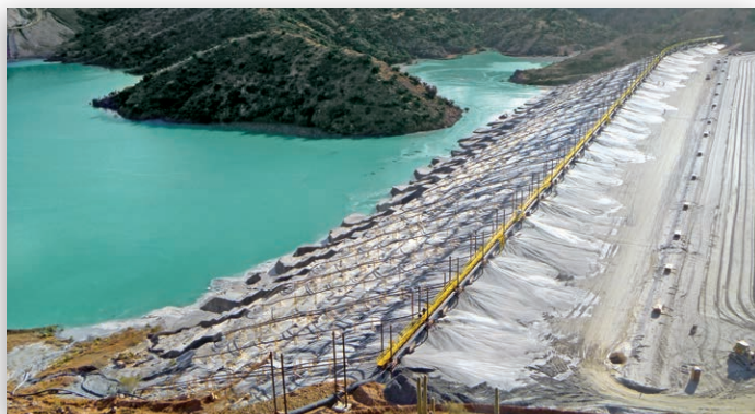
The Upper Mammoth Tailing Dam in Bagdad, Arizona is an expansion to the original dam built in 1985. The dam, constructed using the centerline method, will provide for up to 18 years of tailings storage before reaching its maximum capacity.
