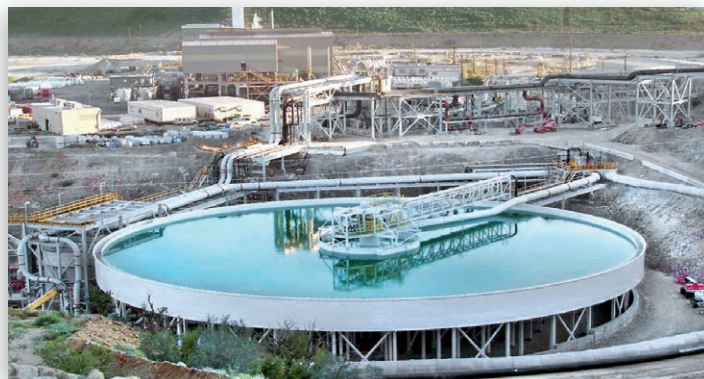
In 2013, the Bagdad mine in Arizona completed construction of the world's largest elevated tailings thickener. The thickener will allow higher volumes of water to be recovered, as well as minimization of seepage and evaporation losses from the tailings storage facility.
